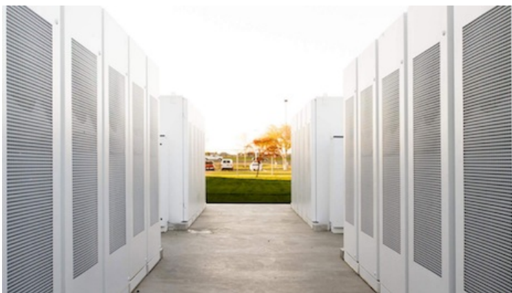
Example of Tesla Powerpack, courtesy of Tesla Motors
